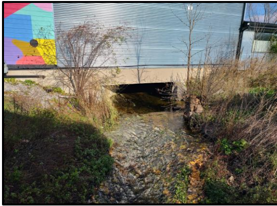
Figure 3-20: Image of Concrete Culvert Under Existing Drake Motor Inn Building Looking North
