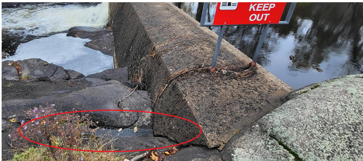
Figure 3-4: Seepage Points Downstream of Overflow Weir
