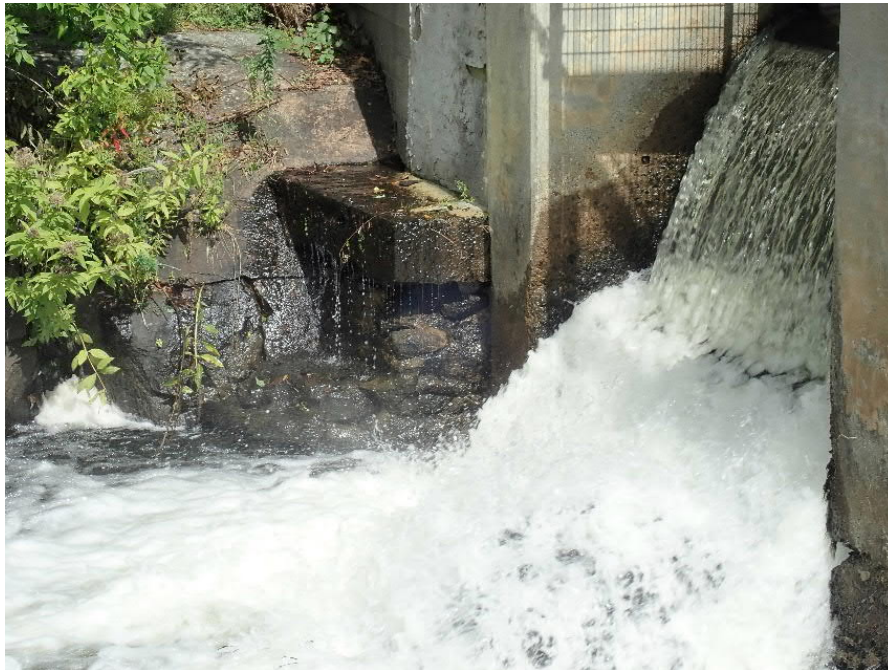
Figure 3-3: Undermining of the Right Wingwall Leveling Slab
