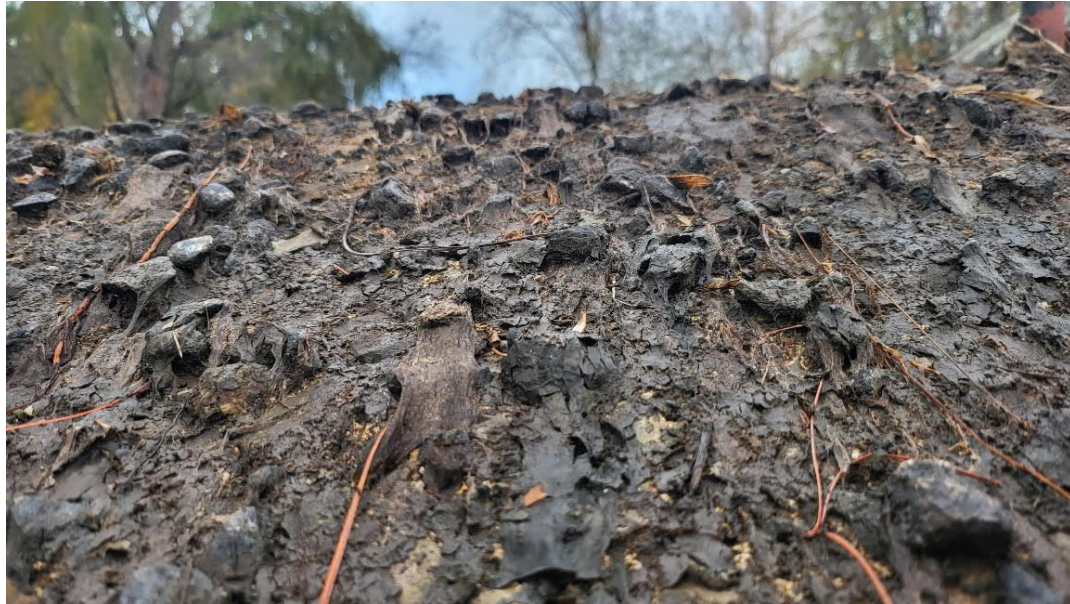
Figure 3-2: Exposed Aggregate on the Overflow Weir
