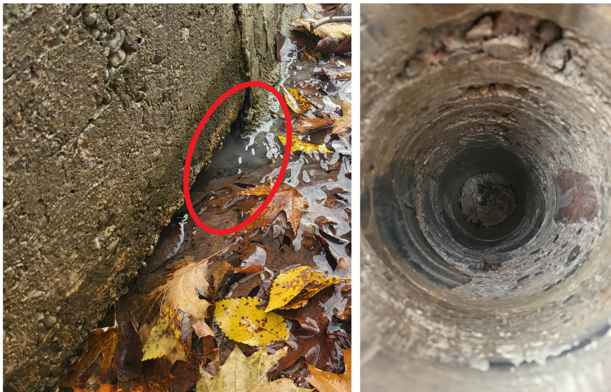
Figure 3-1: Slurry Deposit Downstream of Core Hole 1, Internal View of Core Hole 1
