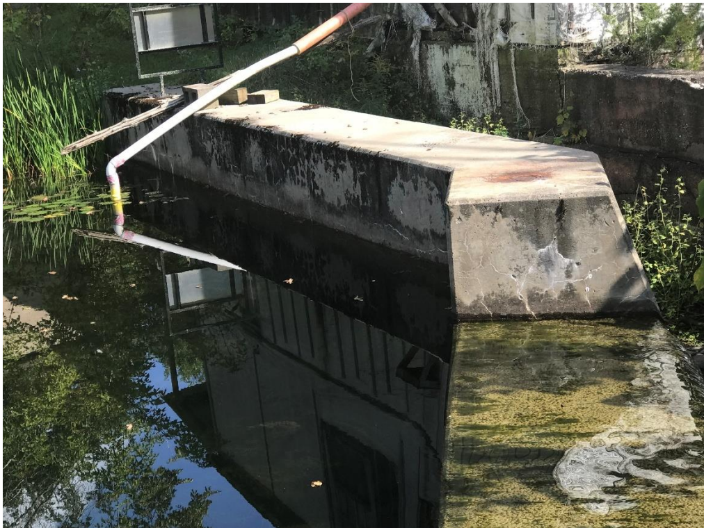
Figure 3.2: Lower Arden Dam, Left Crest of Dam and Spillway from ight Dam Crest, 2024
