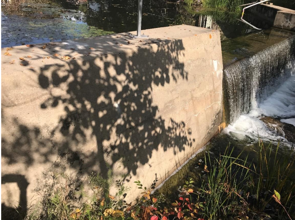
Figure 3.3: Lower Arden Dam, Right Crest and Spillway of Dam from Downstream Right Bank, 2024
