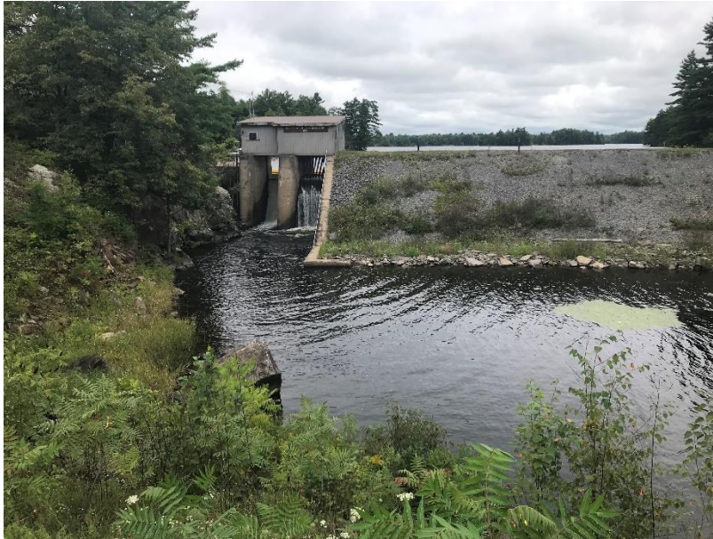
Figure 1: Looking at outlet structure and part of embankment - downstream side of dam - 2023
