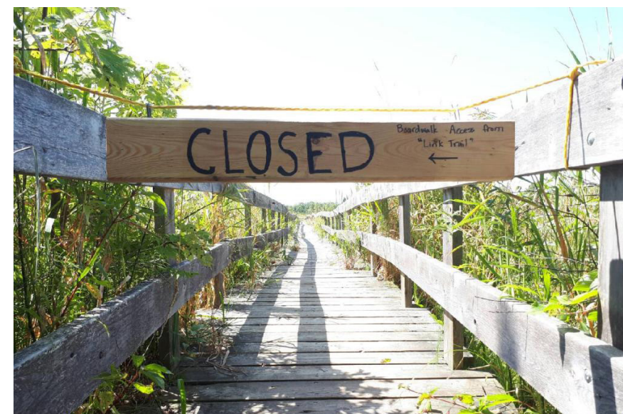
Phase two of the Wetland Ecology Boardwalk re-build project at the Frink Centre.
