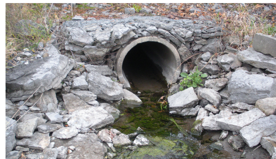
A Stormwater drain with contaminated water.
