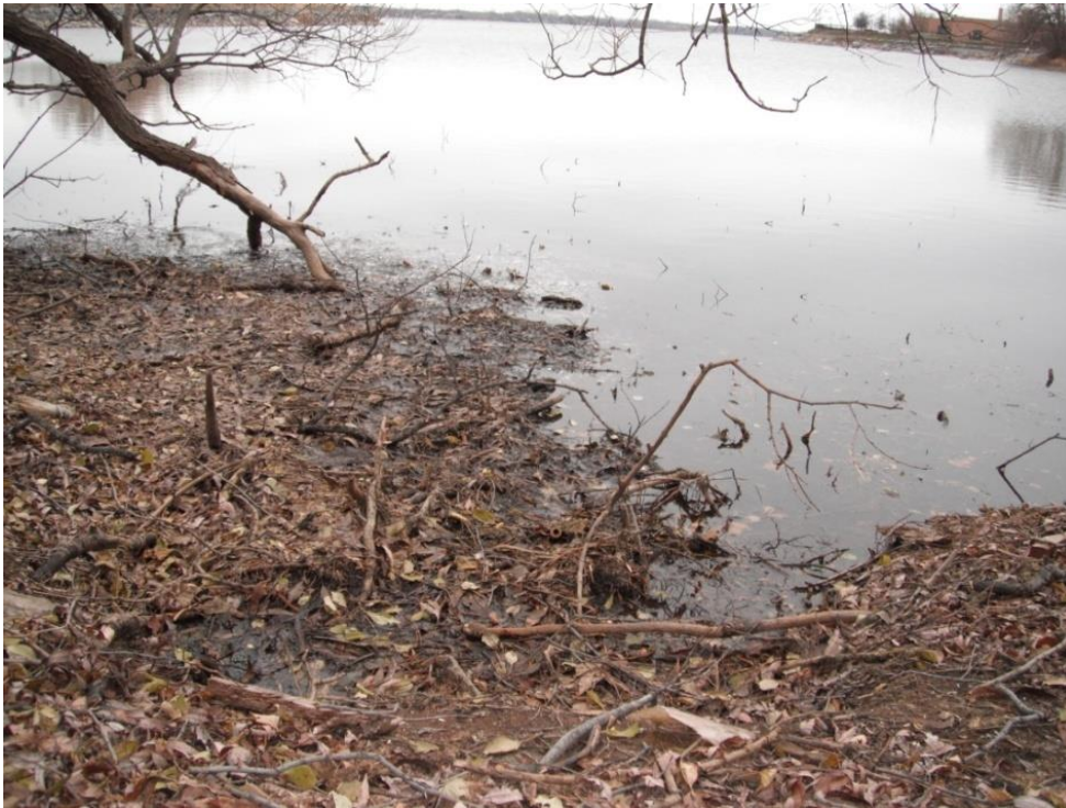
Figure 3: Seep from Zwicks Island Landfill
