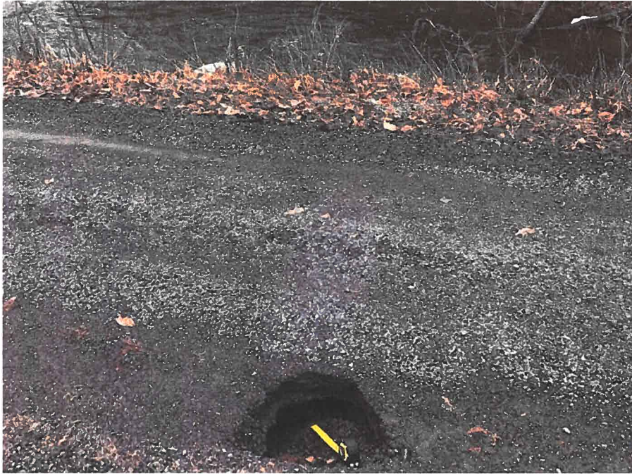
Figure 1 - Thirteen Island Lake Dam sinkhole
