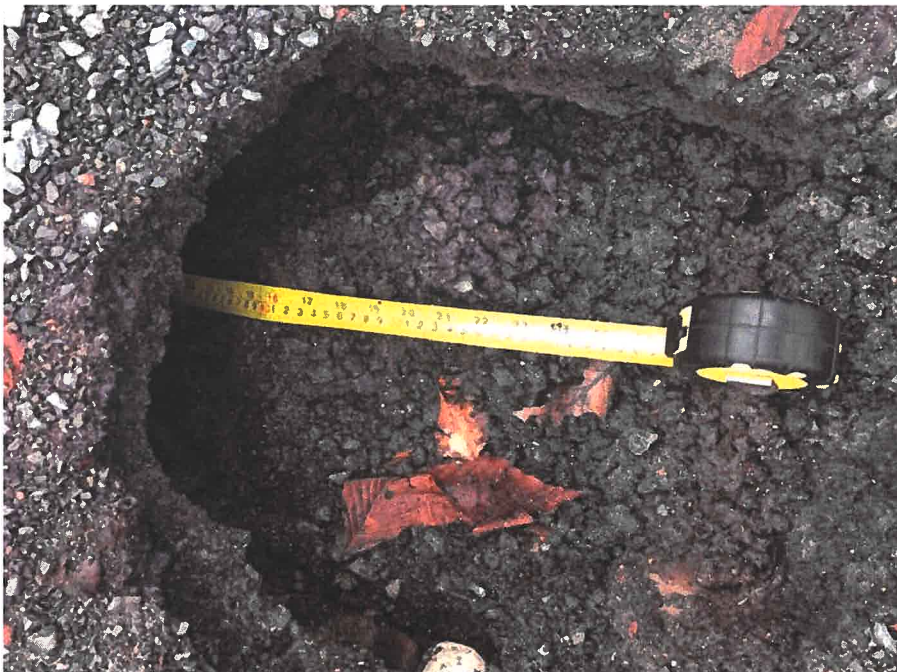
Figure 2 - Sinkhole showing material loss downstream
